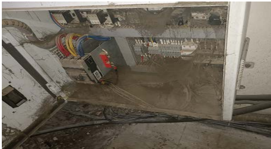
B.Ed. Building, Main Incomer
